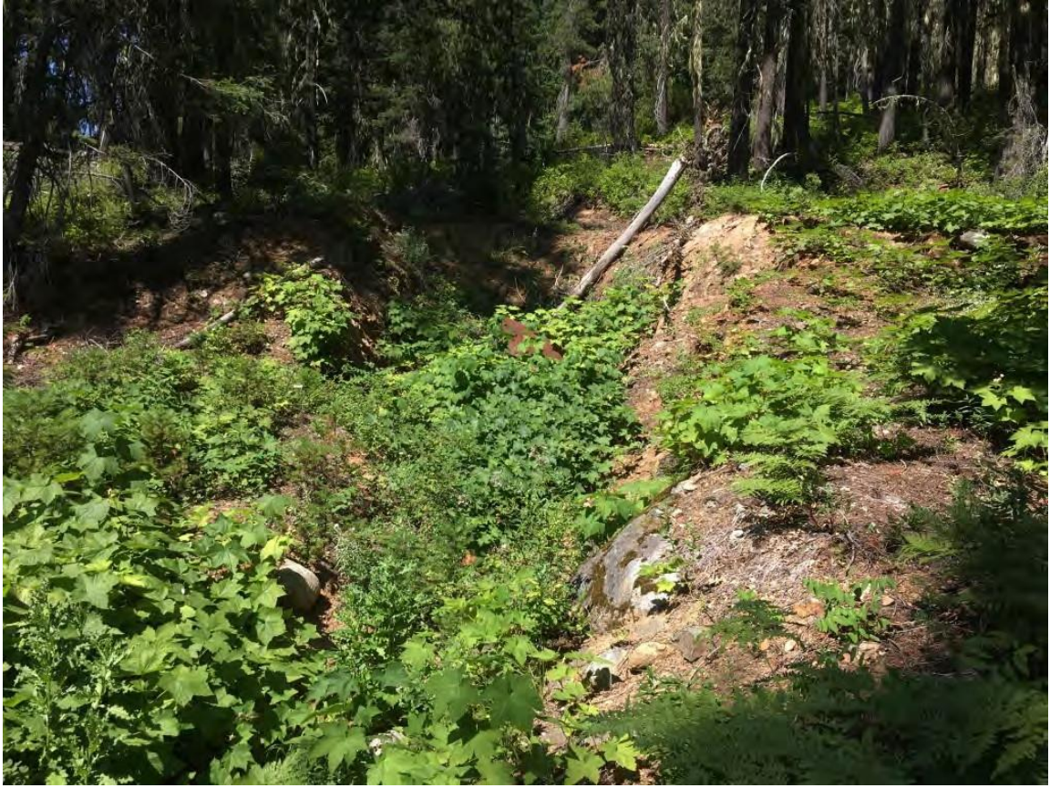
Figure 30: Collapsed portal at the Lower Silver Creek AML site. Portal is located to the south of the tailings pile. Photo taken from mining road looking east. Photo by Scott Kugel, August 2018.
