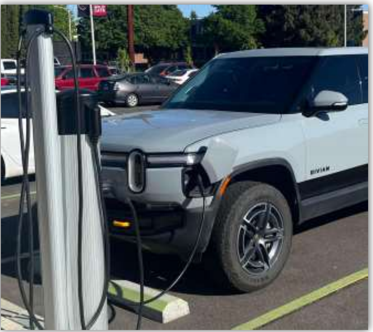
Figure 3. Picture of EV Charging at Nicholson Pavilion
