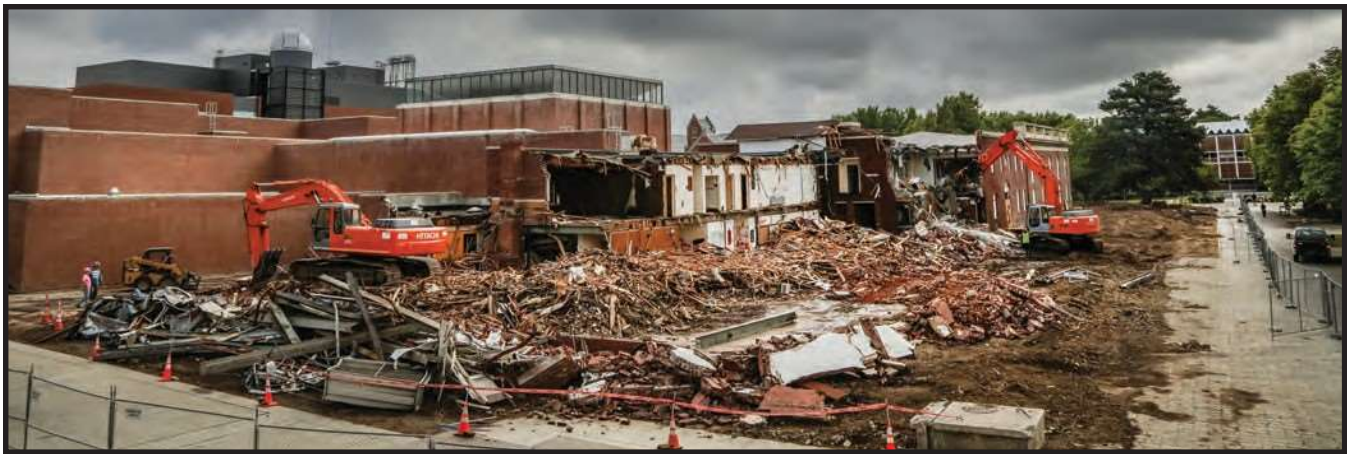
Remodeling and renovating Samuelson began with demolition of part of the original building.
