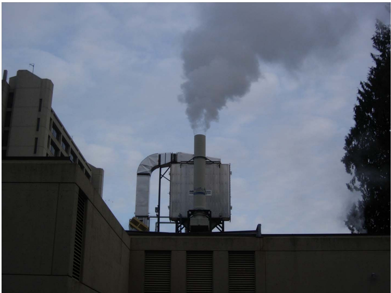
Stack Heat Recovery Unit
